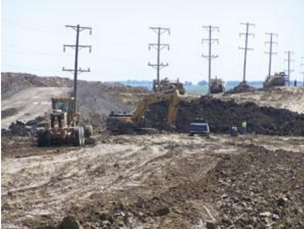
R & G Construction excavated areas to install concrete storm sewer pipes before grading the highway.
