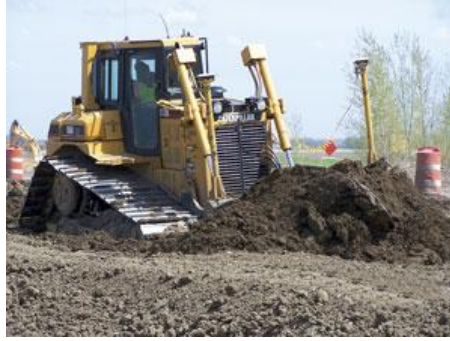
A Caterpillar D6R dozer with GPS moves along the sides of Highway 34 as it levels the road.
