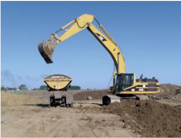
R & G Construction excavated areas to install concrete storm sewer pipes before grading the highway
