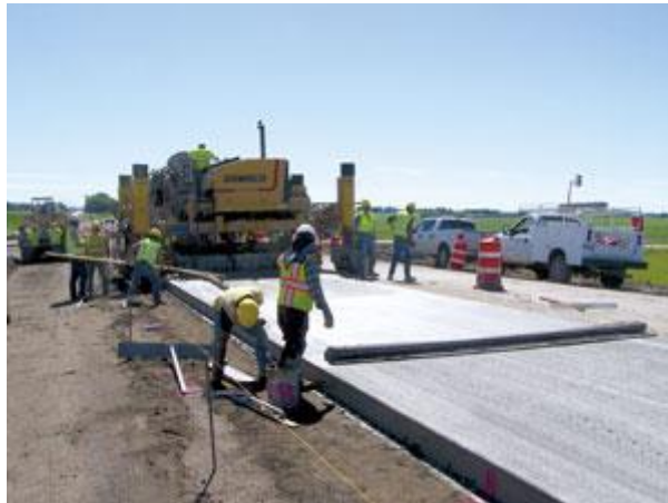
Subcontractor Upper Plains Contracting, Aberdeen, SD, used a Gomaco paver at the west end of the project where Highway 23 was completely graded.
